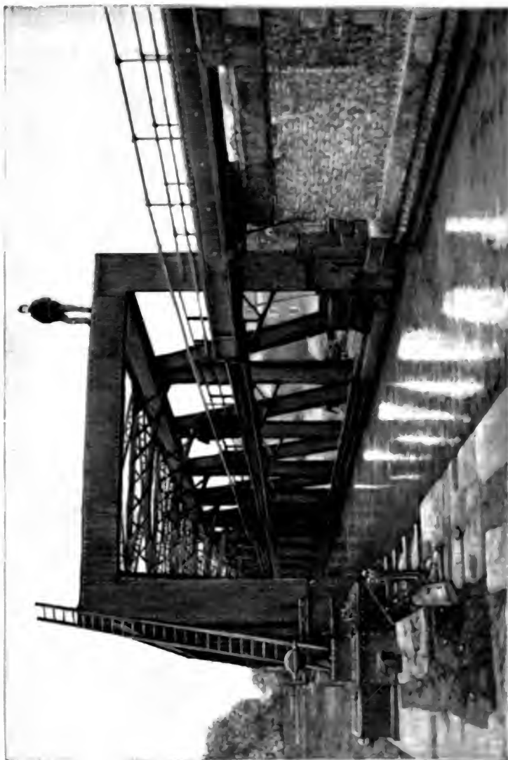
BARTON SWING AQUEDUCT, CARRYING THE OLD BRIDGEWATER CANAL ACROSS THE SHIP CANAL.
